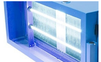
UV ozone lamps to be re installed back in position back into lamp holder and brackets
